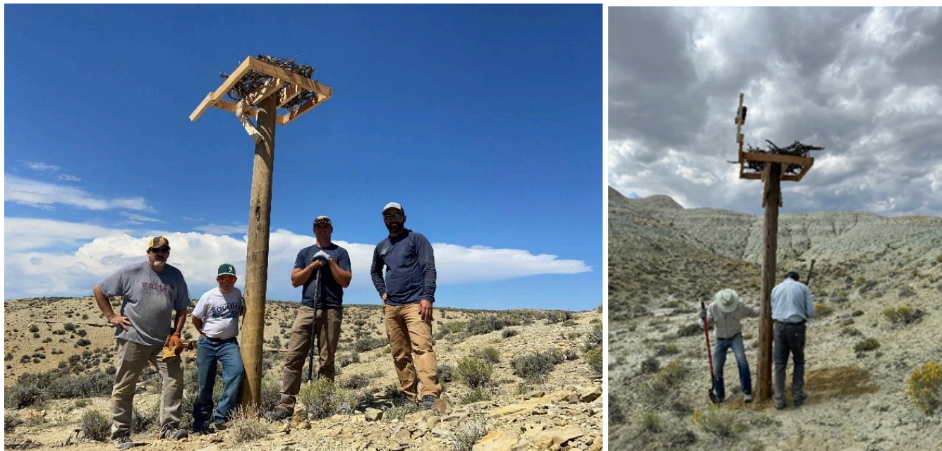
Figure 7. Examples of artificial nesting structures built for Ferruginous Hawks in the NPL area in 2022.
